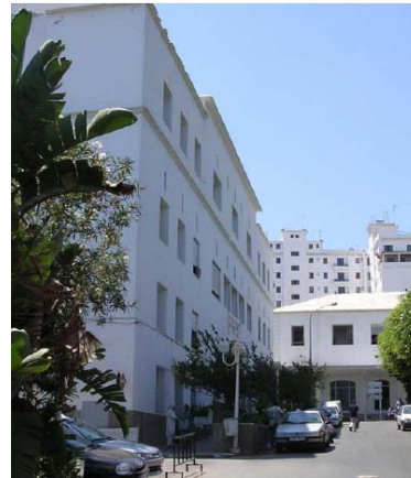
The Hospital Mustapha in Algiers has lost 30% of its rigidity during the 2003 Boumerdes earthquake
