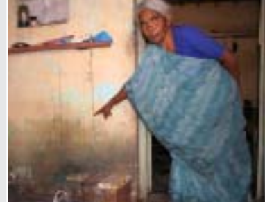
A woman showing the level of water in her house during the floods.
